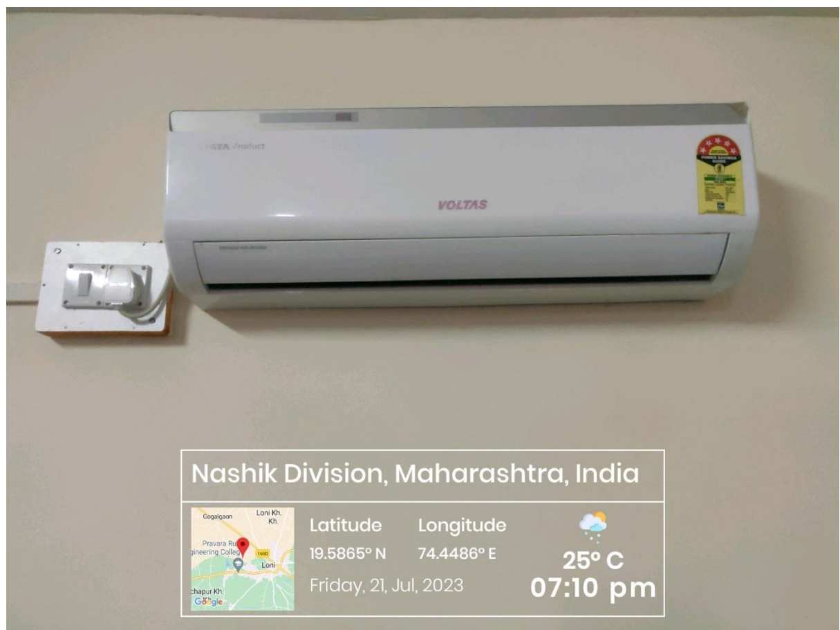
5-star rating AC placed at Board room
