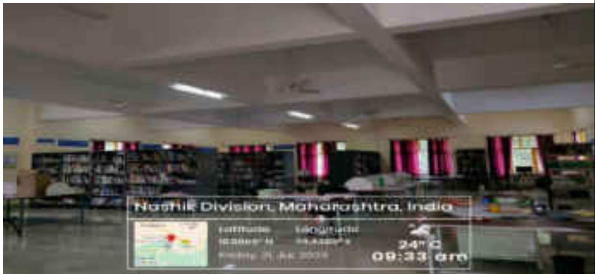
LED lights in Library
