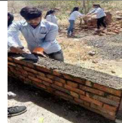
4. Students working collaboratively to get the hands-on experience of masonry wall construction at construction courtyard.
