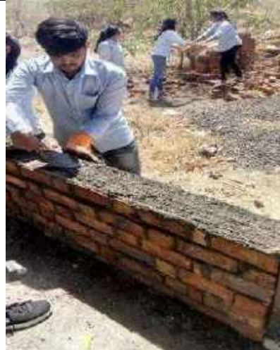
Students placing mortar for the next course of the brick wall in Double Flemish Bond
