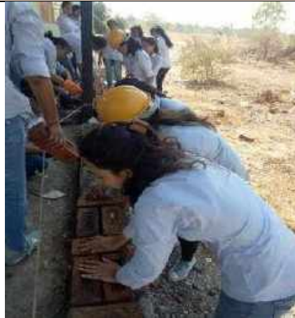
1. Students working collaboratively to get the hands-on experience of masonry wall construction at construction courtyard.
