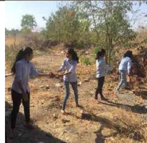
2. Students working collaboratively to get the hands-on experience of masonry wall construction at construction courtyard.
