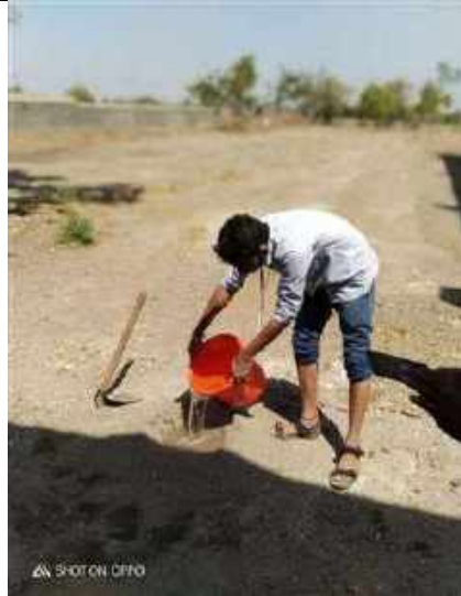
5. Students working collaboratively to get the hands-on experience of masonry wall construction at construction courtyard.
