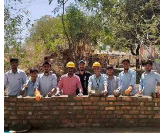
6. Completed Masonry wall in Double Flemish Bond (Result of Participative learning + Experiential learning ) at Construction Courtyard.
