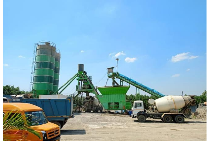
2. RMC Plant with Transit Mixer
