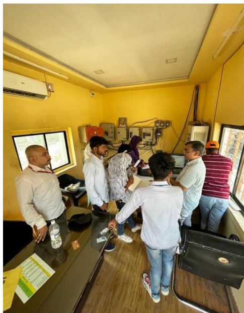
5. Control Room RMC
