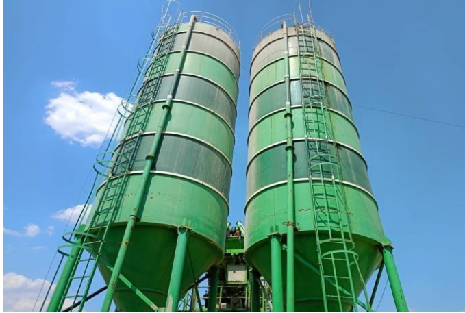
1. Cement and Flyash Storage
